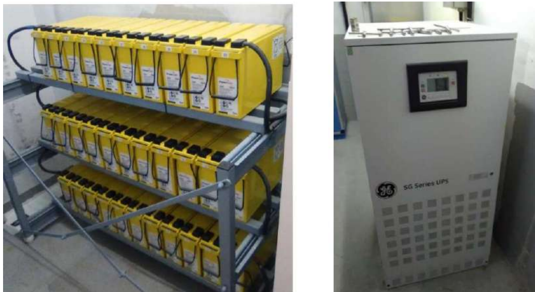
Picture 2: Batteries and UPS
