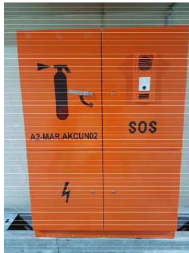
Picture 11: example of a SOS-cabinet
