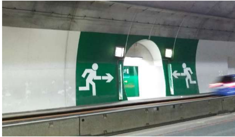
Figure 6: Example of emergency escape route with sliding fire resistant door and proper marking
