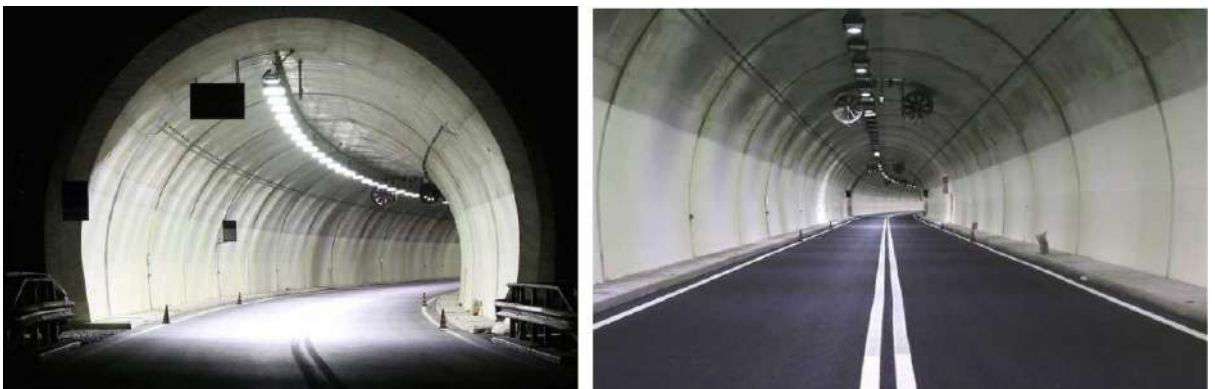
Picture 4: Example of tunnel lighting equipment
