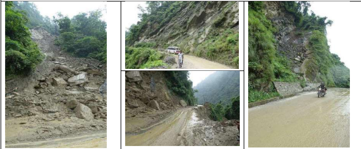
Fig. 5 : Photographic Report – Road General Layout-Steeper and Eroded Slopes
