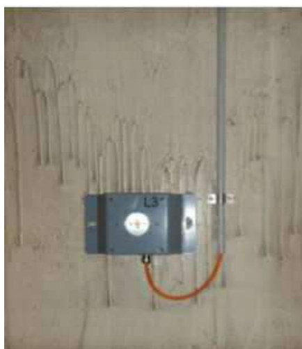
Picture 3: Example of fire emergency lighting
